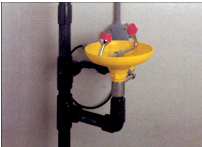
A simple push-type hand-operated valve activates the eyewash unit.
